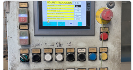
HMI & Control Diagnostics
